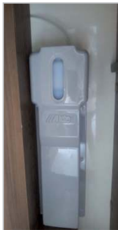
Fig.6.41 - Glycol mixture level
